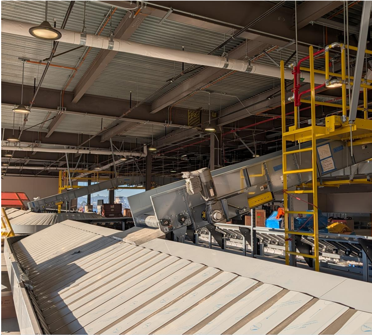
Area D Baggage Handling Systems
