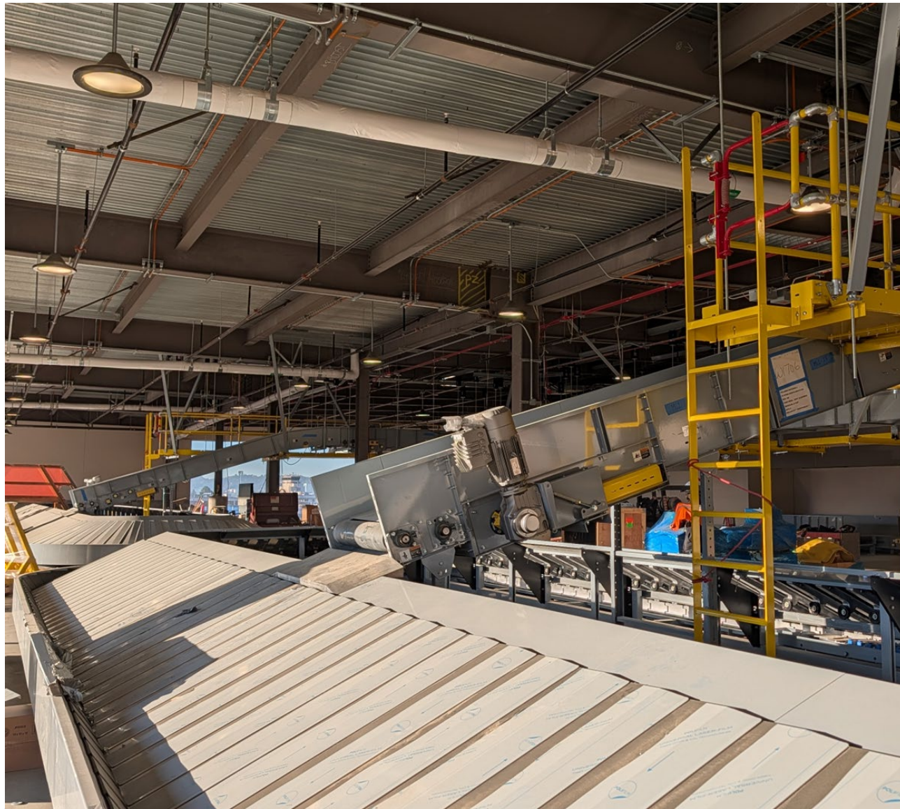
Area D Baggage Handling Systems
